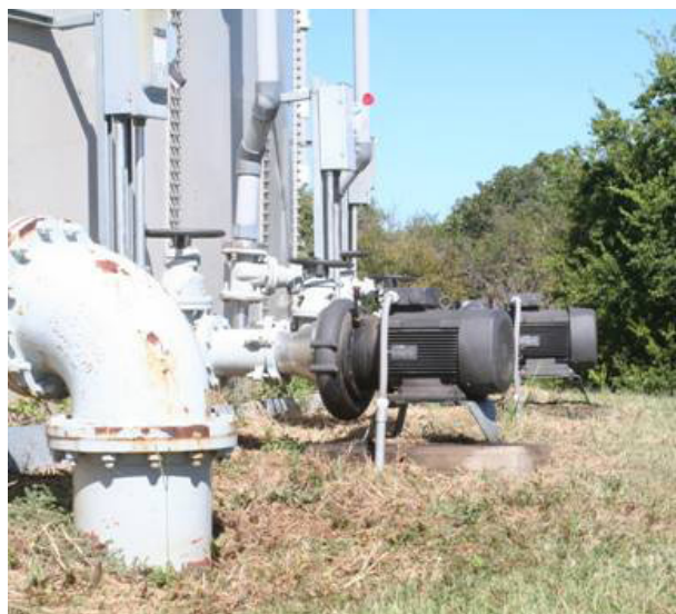
Externally mounted chopper pump aeration system at Gun Barrel City
