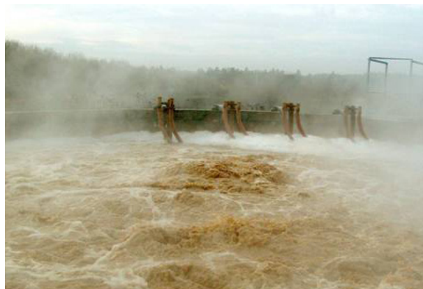
This equipment provides simultaneous aerating and mixing.
